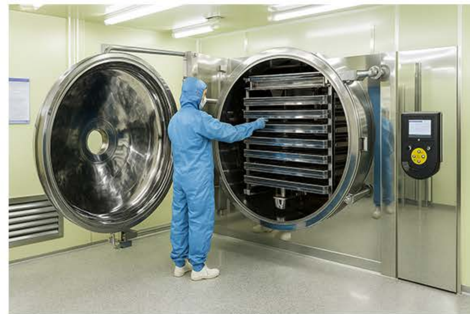
► Freeze-drying processing line
